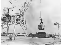
TEST reactor is lowered into deep pit by crane on site. The deep pit is shielded.
